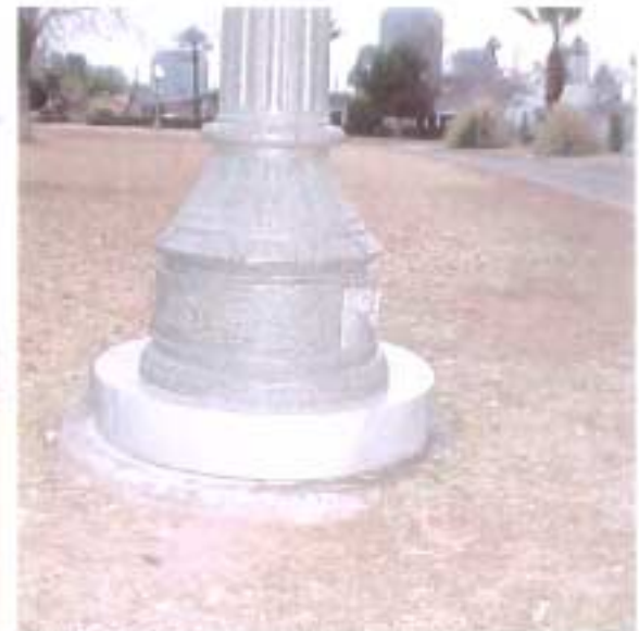
Photo 29. Base installation. The sheet metal bases are easily damaged.
