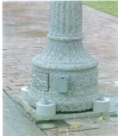
Photo 19. Heritage Square. Inappropriate installation method with visible mounting bolts.
