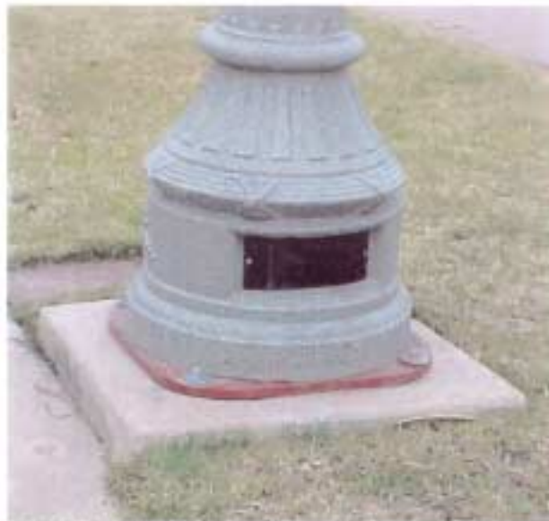
Photo 27. Adapter plate at base. Concrete pole replaced historic metal pole. Looks out of place along Palmcroat Drive NE.
